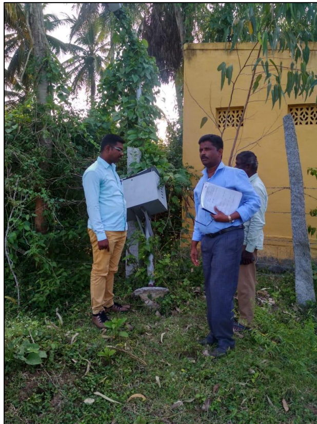
Photo 25: Community benefit, Maddur range, Mandya division, Mysuru circle Damaged solar street light
