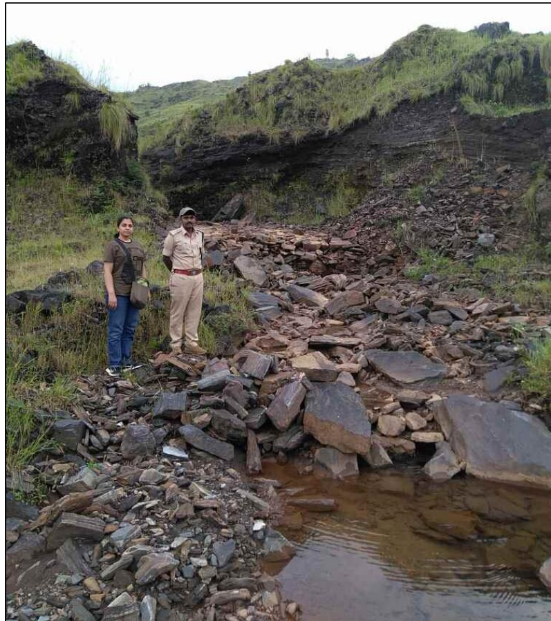
Photo 27: Gully checks damaged, Kudremukha WL range, Karkala WL division
